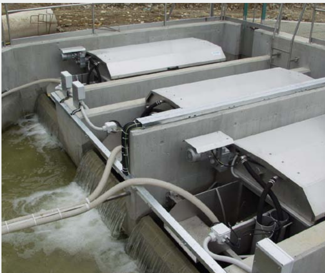
Custom made battery channel installation. Simple to maintain during operation.
