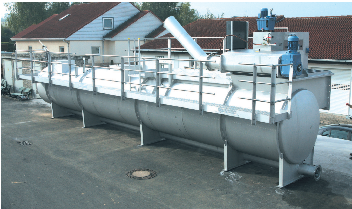
W+F cylindrical grit separator compact system for inlet flow Q = 280 l/s
